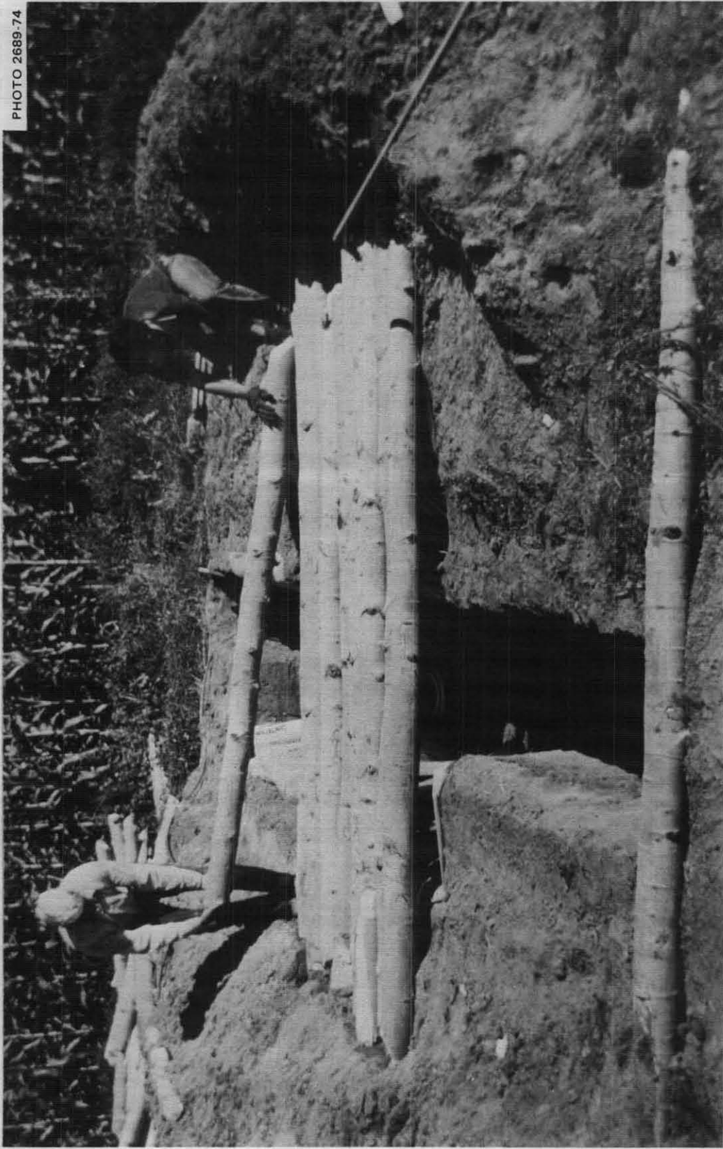
Fig. 4.7. Placing the 9-ft roof logs, all 2 ft off center, over the 3½-ft-wide main trench. A shelter in firm earth such as this, with 9-ft roofing logs positioned 2 ft off center, would enable the builders to widen their shelter to a 5½- or 6-ft width and to deepen it to standing height. If their home and community were destroyed, the family could live in such a rainproof dugout for months, if necessary, while minimizing their radiation doses and being more comfortable, in cold weather, than if living in a tent or shack.
